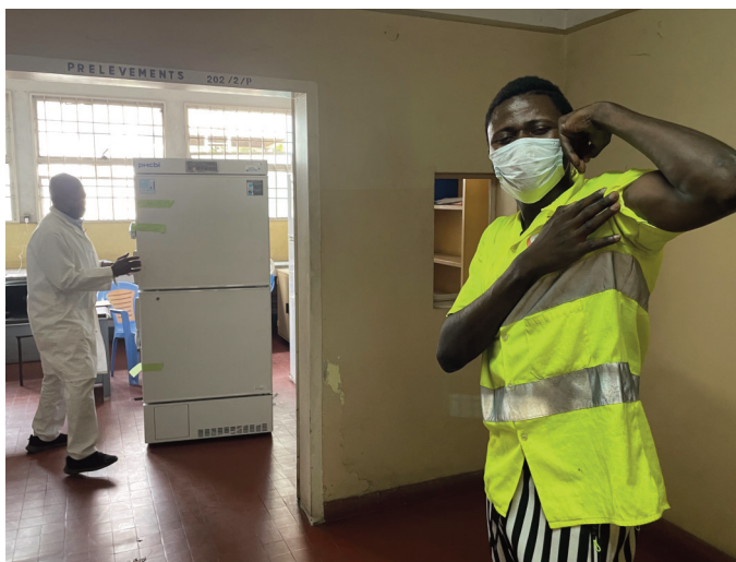
Installation of PHCbi equipment. National Institute of Biomedical Research, Democratic Republic of the Congo
